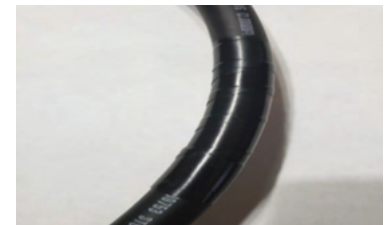
IMAGE B – ELECTRICAL TAPE IS NOT APPROVED
