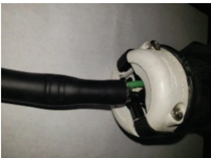
IMAGE E – CORD NOT IN RESTRAINT IMPROPER INSTALLATION
