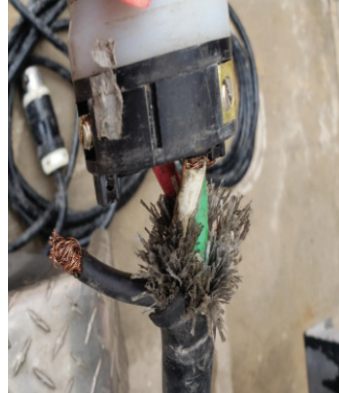
IMAGE H – RESULT OF IMPROPER INSTALLATION
