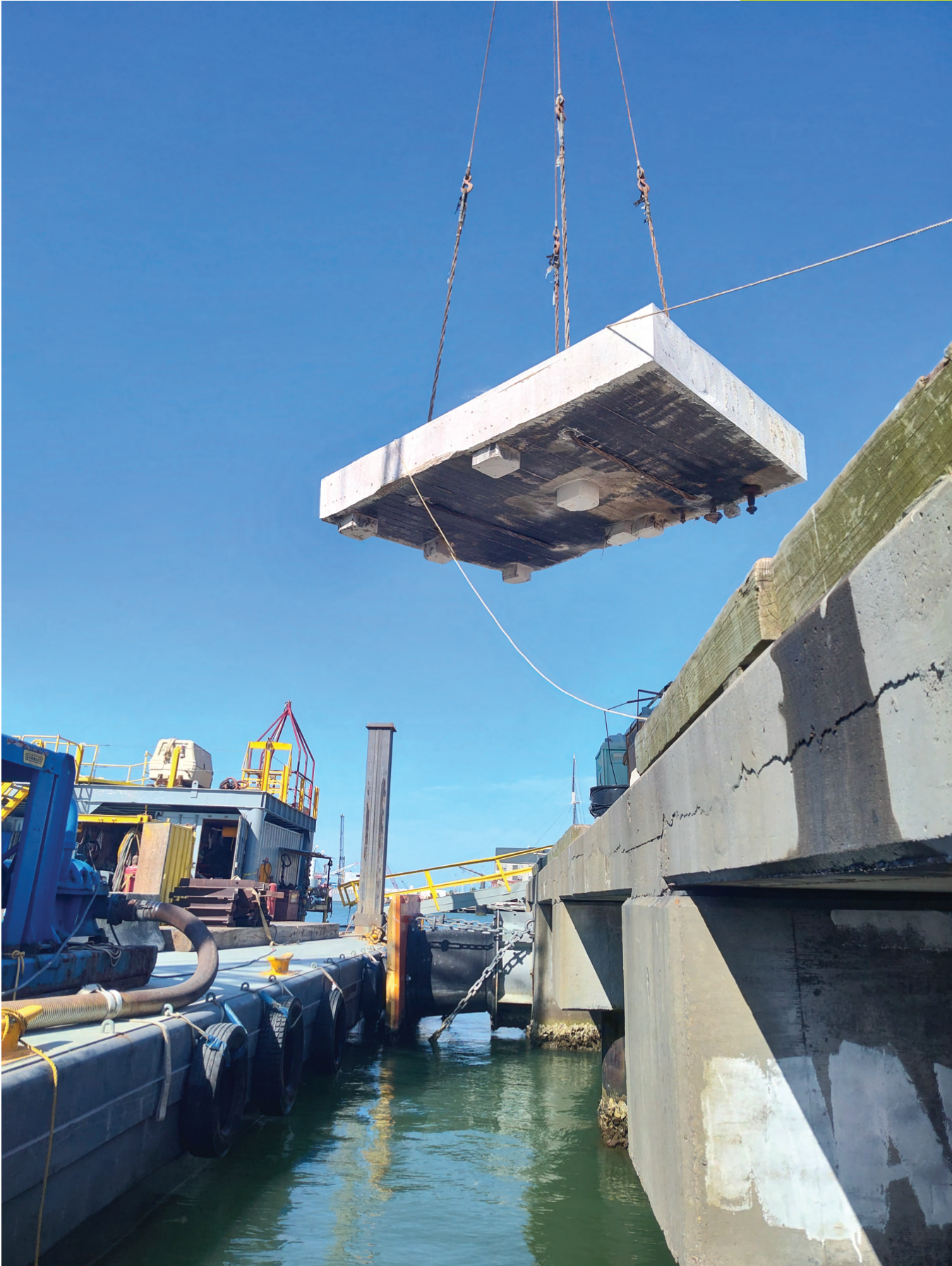
The largest portion of concrete deck removed measured 240-feet long by 12 to 14-feet wide, with varied depths up to 24-inches thick.
