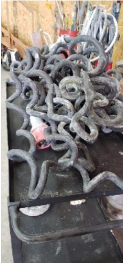
IMAGE D – OVERHEATED DUE TO CORD REEL
