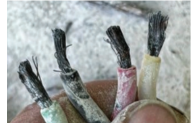
IMAGE A – CORRODED CONDUCTORS
